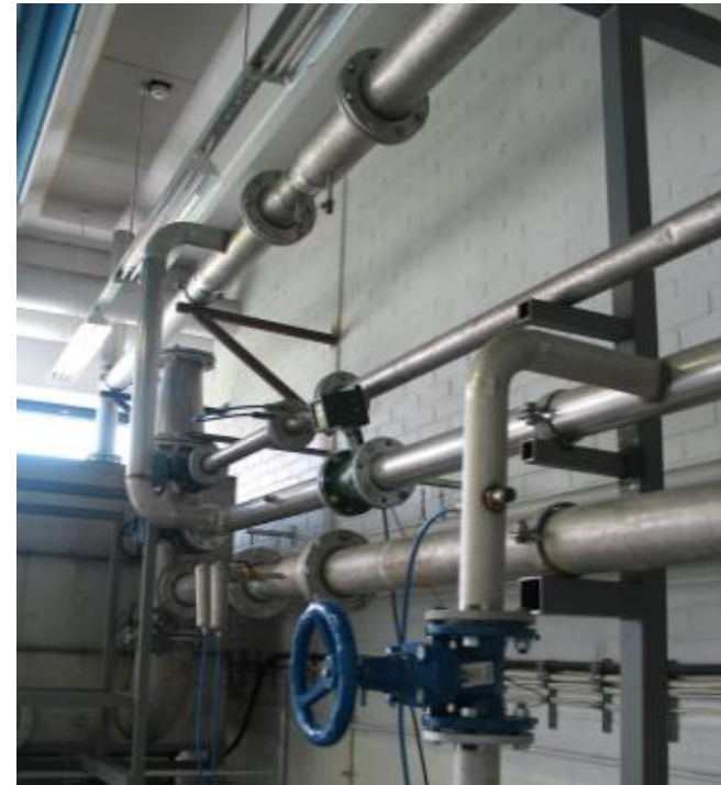
Figure. Old pumping system laboratory in LUT
